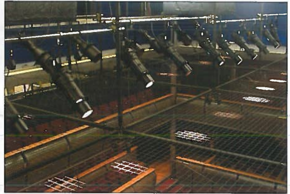
Left, chief technician Charlotte Walker and technical manager Phillip Dexter; above and below, lighting grid shots from Circus 1
